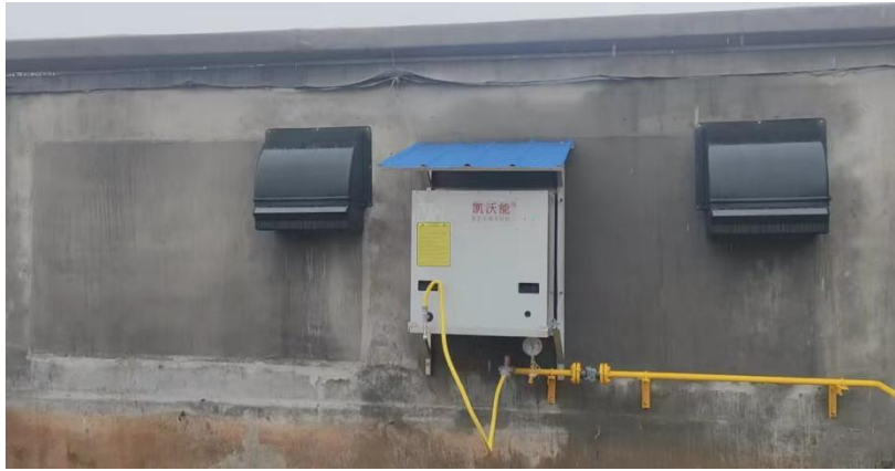
KWDHVSO70 unit installation
