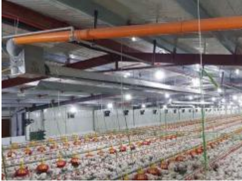
Overall broiler-house interior and radiant heater layout
