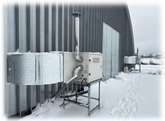
Close-up view of the heater unit
