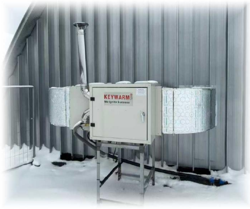
Close-up view of the heater unit
