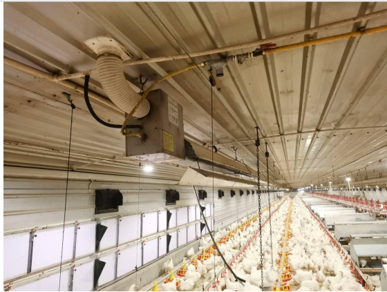
LTSA35-18 close-up and along-wall installation scene
